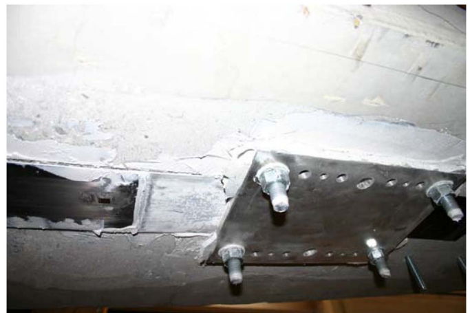
Fig. 6. View of the secondary failure due to sliding of the CFRP laminate under the anchor plate
