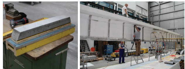
Fig. 7 Concrete bolsters and shear strengthening with EB-CFRP sheets wrapped entirely around girder.
