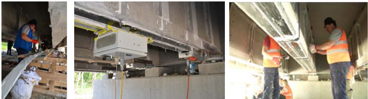
Figure 9. Application of prestressed CFRP laminates with the gradient method and shear strengthening
