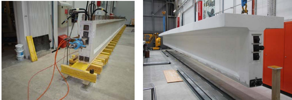
Figure 3: Posttensioning of the concrete girder with steel cables (left) and the full T-section girder after slab concreting(right) [3].
